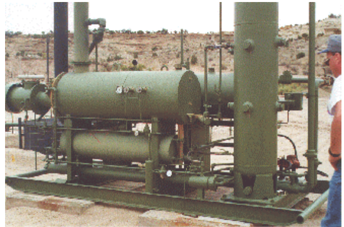
Figure 1: Gas-Fired Dehydrator Boiler in Field
